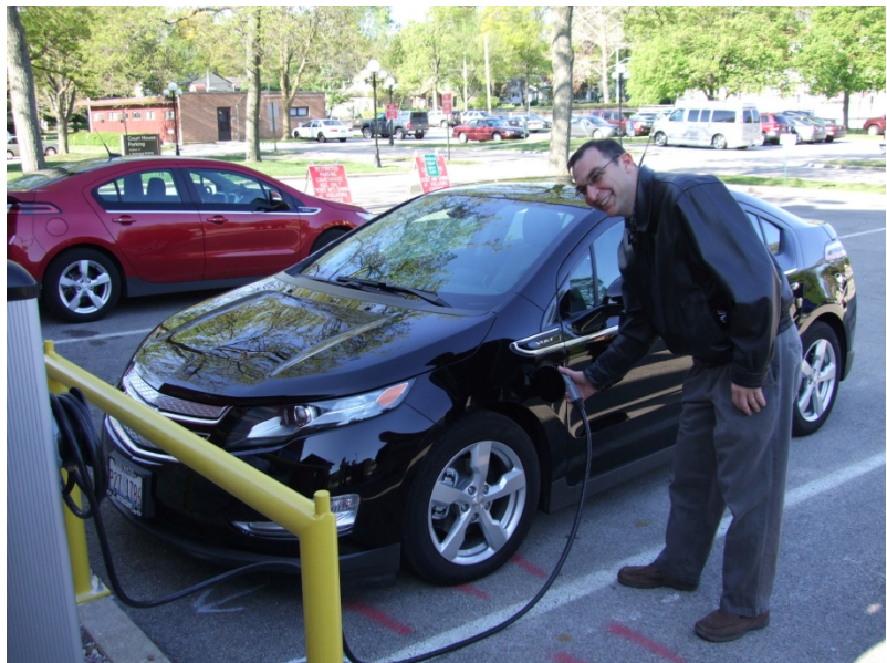
ELECTRIC VEHICLE CHARGING STATION INSTALLED AT KANE COUNTY’S THIRD STREET COURTHOUSE, GENEVA, IL
