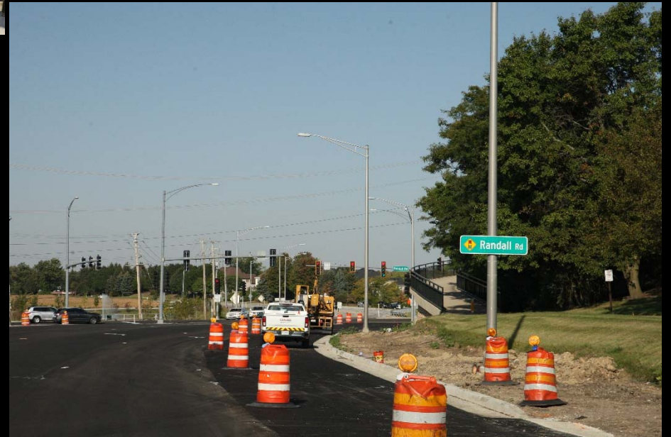
Crews auger holes for new guardrail posts and rail for a new right turn lane on westbound Silver Glen Road at Randall Road
